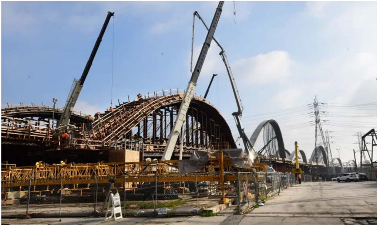
Construction workers pour concrete on the arches for the Sixth Street Viaduct project in Los Angeles. | Photo by Frederic J. Brown/AFP via Getty Images
